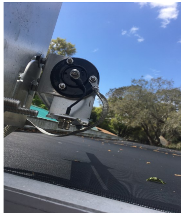
Tilt-over antenna mount with Braid going to the pool cage.
